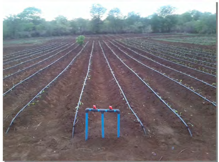
Figure 2: Drip irrigation facility at Community Centre
